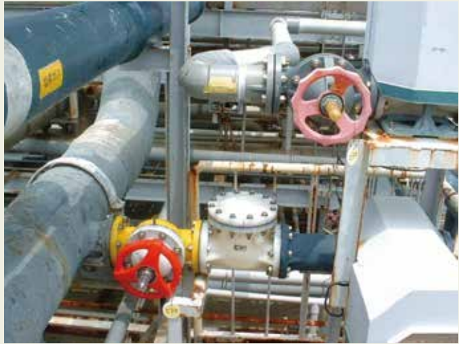
⋈ PVDF swing check valve installed horizontally at a chemical plant and has been working for more than 20 years.
