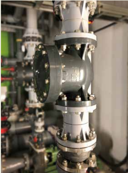
⋈ Vertically-installed swing check valve at an aquarium in Japan.
